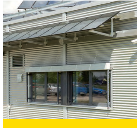
Facade cladding with solar modules providing solar control on a building belonging to the Max Fuss company in Berlin
